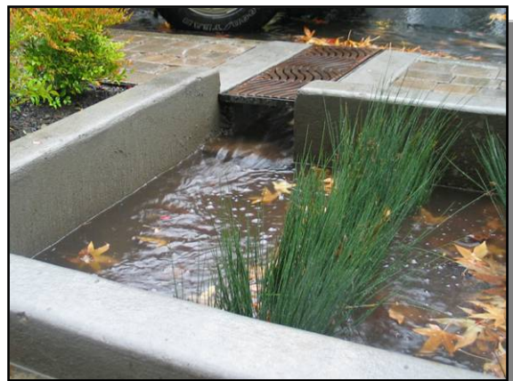
Rain gardens and infiltration zones improve the quality of water leaving the site
